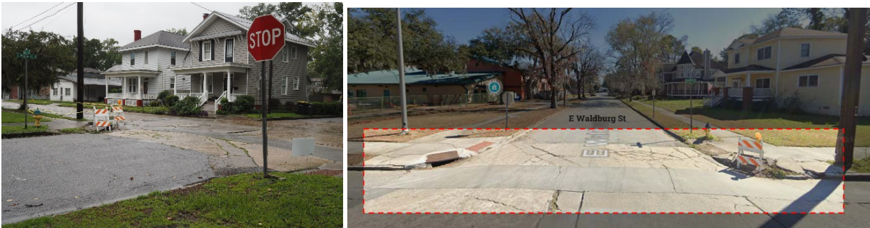
Images. Broken curb cuts and cracked road surfaces on the street hinder smooth movement, reducing accessibility for pedestrians. Photo by EC and Google Streetview, 2022
