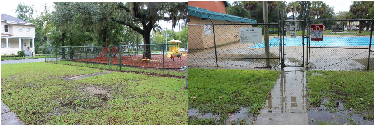
Images.. The access to the children's area is not ADA friendly (left) just like the pool access (right). Photos taken by EC, 2022.
