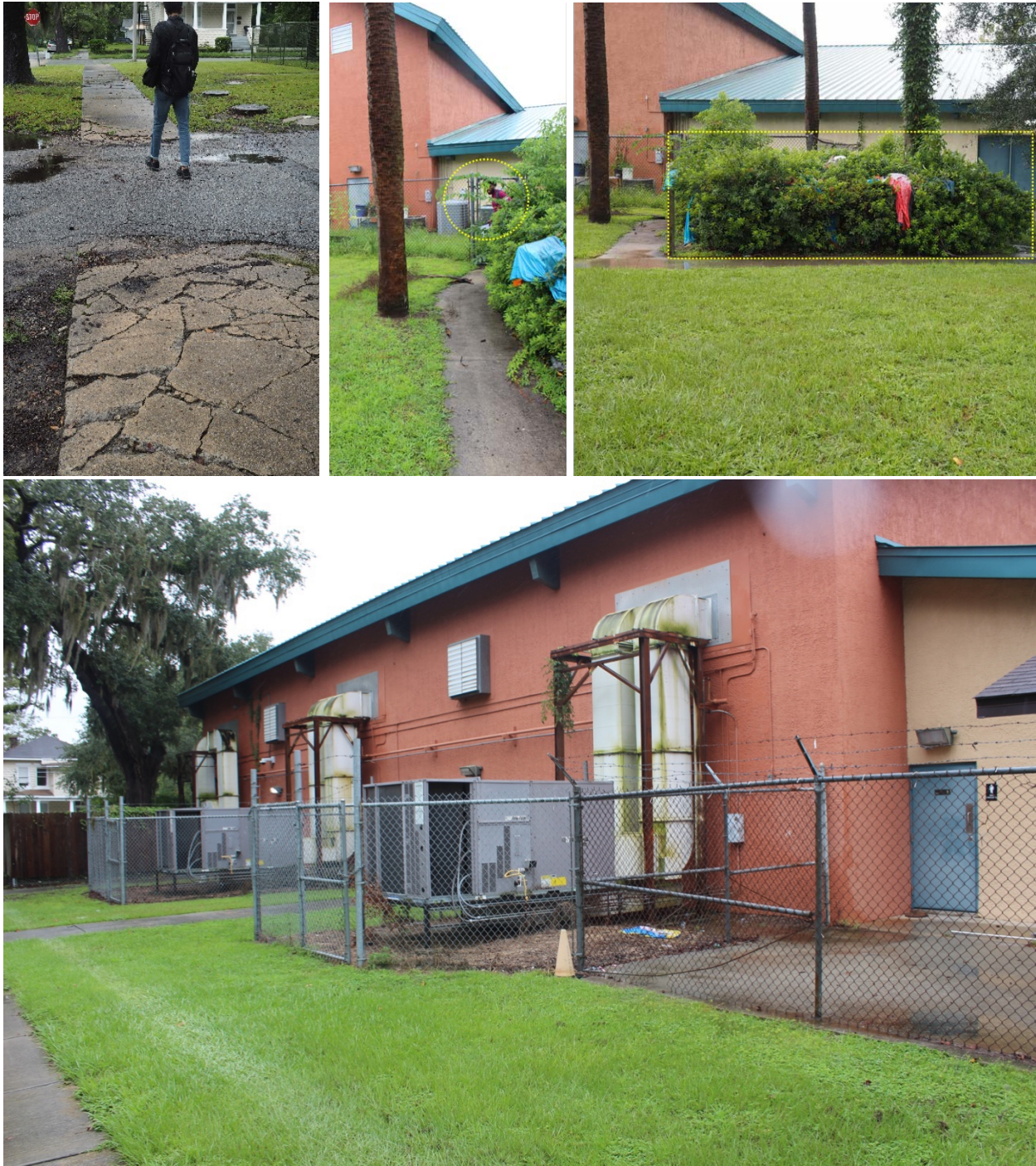
Images. The backside of the community center and community garden area by the pool are poorly maintained. The sidewalks have cracks and broken slabs in multiple places (middle). The park signage is obstructed (right). Photos taken by EC, 2022.
