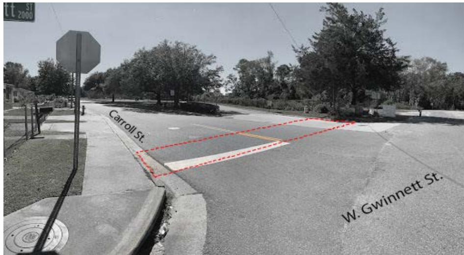
Image. The sidewalk along West Gwinnett Street bends to follow Carroll Street. Note the narrow width, poor maintenance, and lack of ADA-compliant design features. There are also no crosswalks provided to access the park. Photo by EC, 2022
