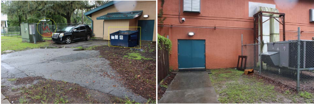
Images. The back side of the W.W. Law Community Center directly fronts E Waldburg Street with utility doorways, exposed HVAC units, and wire fencing along the entirety of property's southern boundary. Photo from EC 2022.
