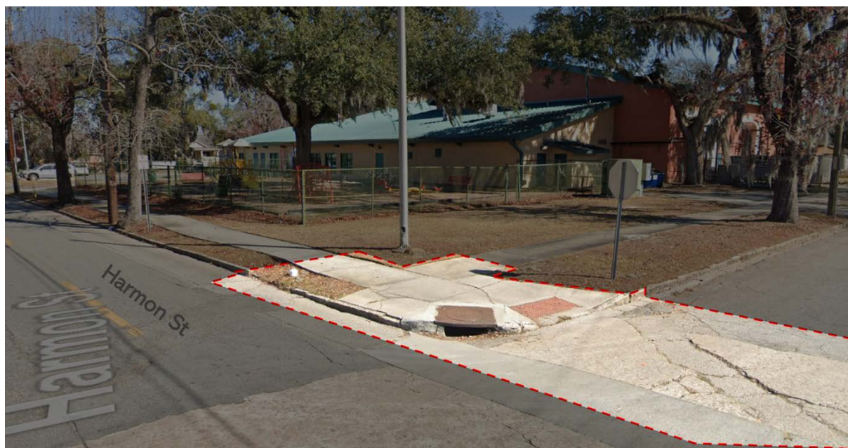
Image. Improperly done curb cuts and cracks on the crosswalk area of road surface. Photo from Google Streetview, 2022
