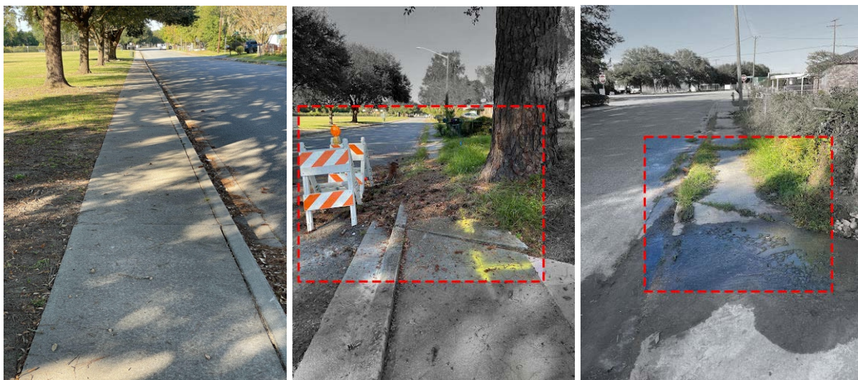
Images. A sidewalk along the park on Carroll St (left); sidewalks requiring maintenance due to uneven surface (middle); water seeping onto the sidewalk from open pipe connection (right). Photo taken by EC, 2022.
