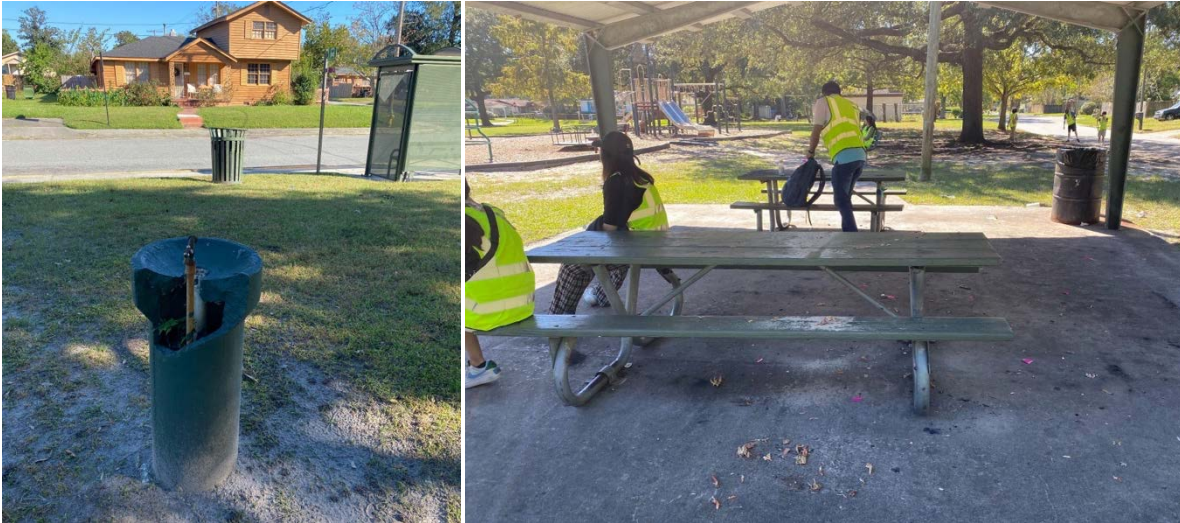
Images. Condition of the water fountain (left) and litter inside the gazebo (right). Photos taken by EC, 2022.
