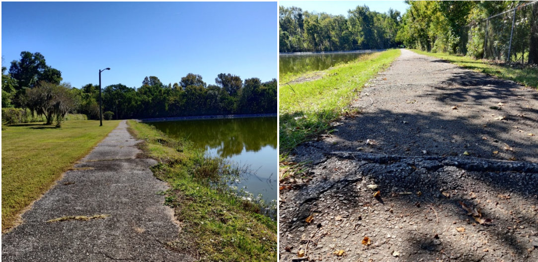
Images. Undefined edges of the walking path (left); cracks in the pavement (right) Photos taken by EC, 2022.
