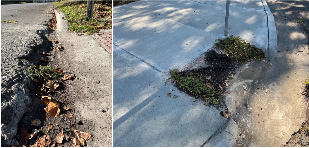
Image. Poorly maintained curb cut at the western corner of Cann Park on 45th Street (left) and uneven curb cut (right). Photo taken by EC, 2022.
