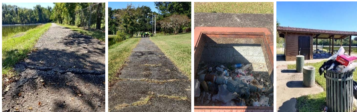
Image. Poor quality of pavement with cracks and in-growth in multiple locations (left); trash and litter around the park (right). Photos taken by EC, 2022.
