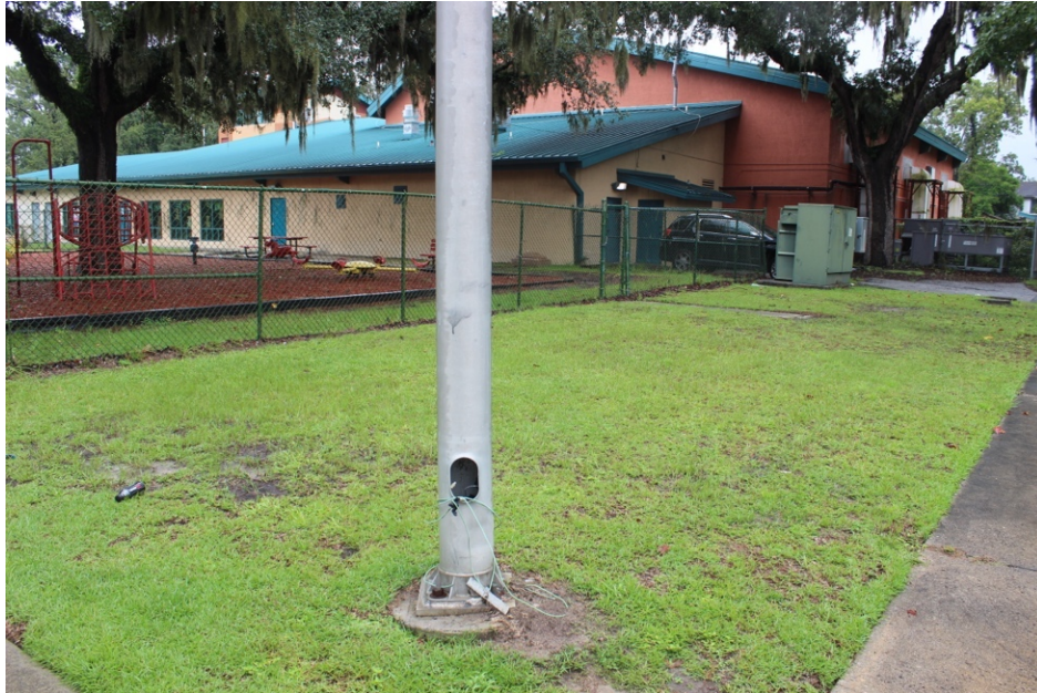
Image: A missing cover and strewn wires on a light pole at W.W. Law Park. Photo taken by EC, 2023
