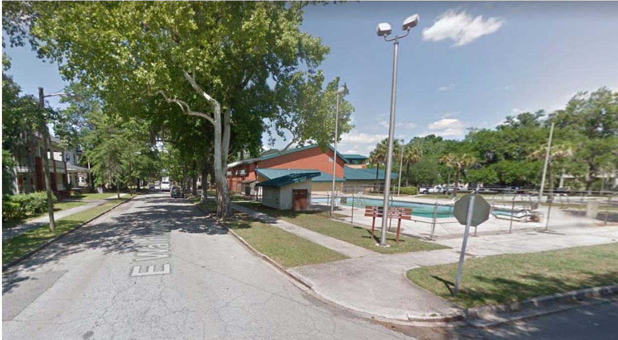
Image. Broken curb cuts and cracked road surfaces on the street hinder smooth movement, reducing accessibility for pedestrians. Photo by EC and Google Streetview, 2022
